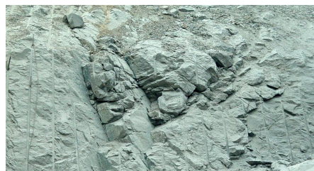
图 2 组合块体松弛变形 Fig.2 Unloading deformation of rock blocks
