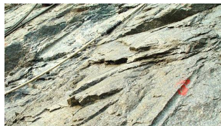
图 3 小湾拱坝右岸建基面岩体表层“葱皮”松弛现象 Fig.3 Looseness phenomenon in shallow rock mass of right abutment of Xiaowan arch dam
